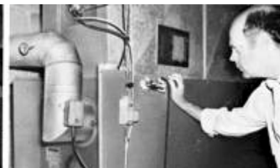
Taking over-fire draft reading with Inclined Draft Gage held by Magneclips (included). Not Stack Thermometer secured by holder.
